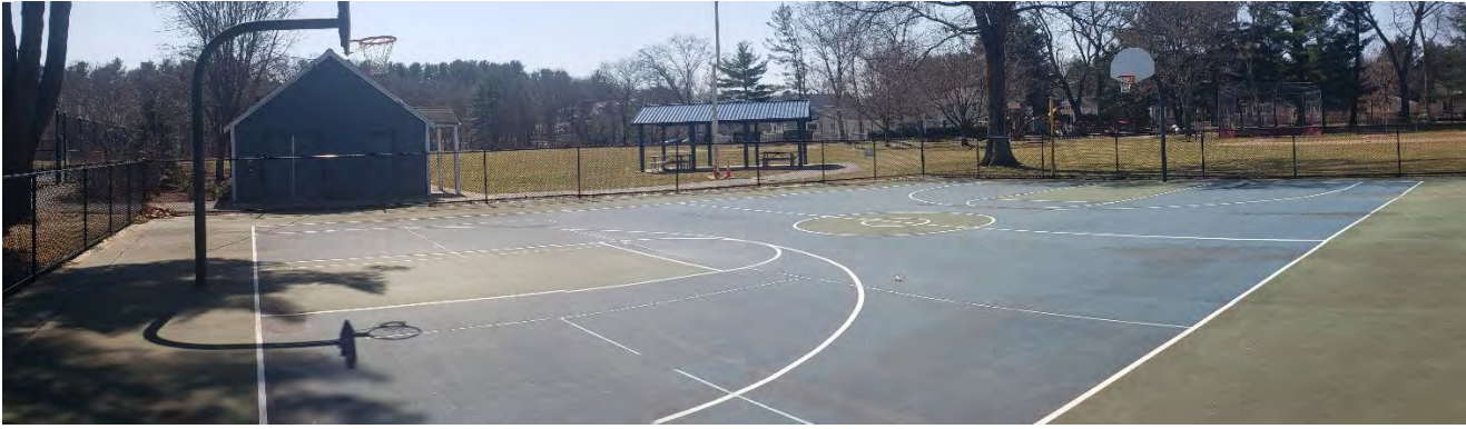
Basketball Court #2. Some fading and cracking.
